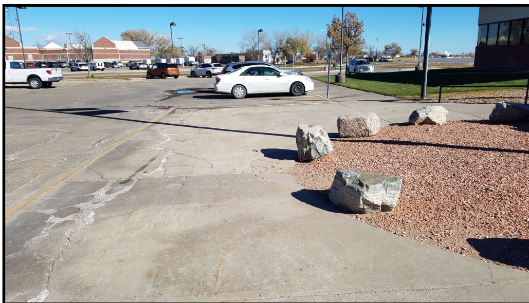
Main Entry – Damaged Concrete
