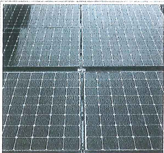
Solar panels on roof of home
