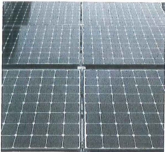
Solar panels on roof of home
